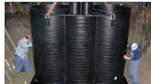
Utilization of the monolith extraction pit for the installation of two 2-fold containerized lysimeter stations
