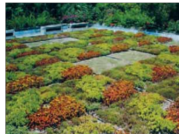
Lysimeters integrated in the green roof construction
