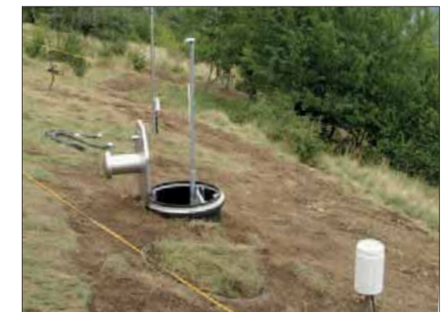
Hillside lysimeter at Sierre/Switzerland direct after installation
