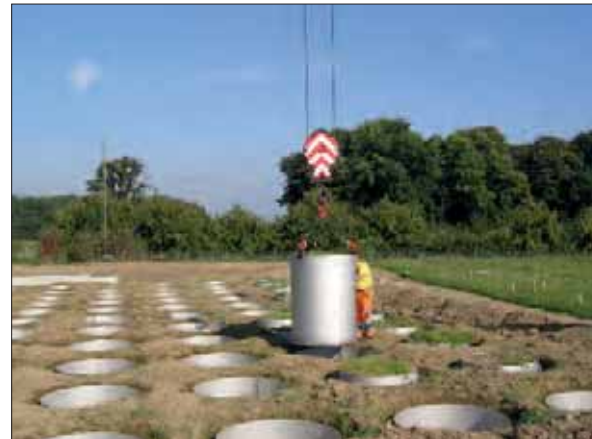
Stainless steel lysimeter vessel is installed at the lysimeter station
