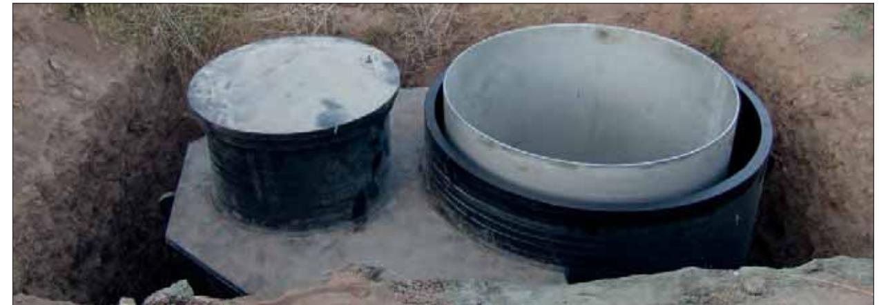
Containerized Lysimeterstation during the installation works
