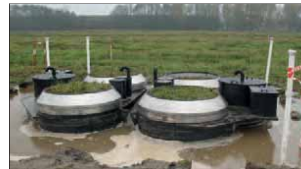
Lysimeter stations after the installation of the waterproof collars and deinstallation of the groundwater lowering
